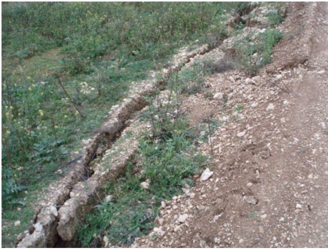
Fig. 3 Tension crack developed in August 2006 that defines the upper boundary of the slid mass
